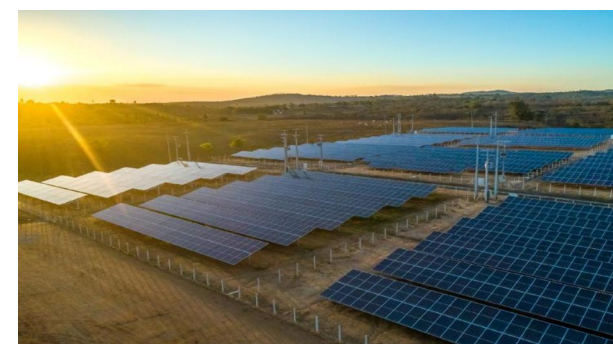
Setta PV Plant
