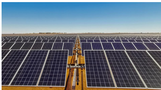
Kimberly Droogfontein PV Plant
