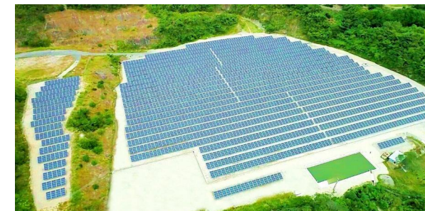
Kanzaki PV Plant
